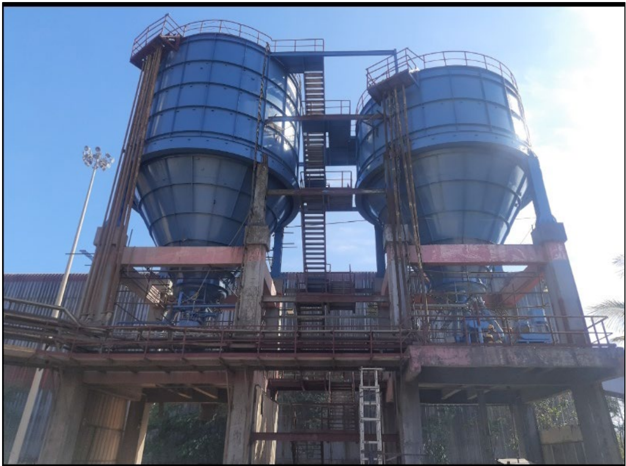
Photographs of Silo (Bottom Ash and Fly Ash)
