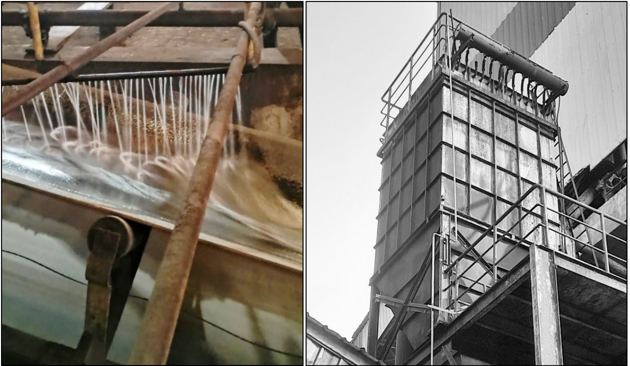
Photograph of the Water Sprinkler System and Bag filter
